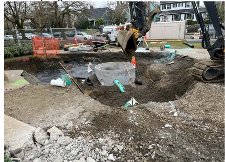
Installation of new storm system manhole on south end of the site
