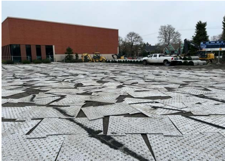
Existing shock padding following removal of artificial turf from south end of field
