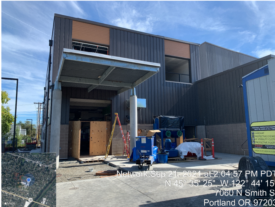
West side of RHS P4 addition showing CTE overhead door opening and dust collection equipment.
