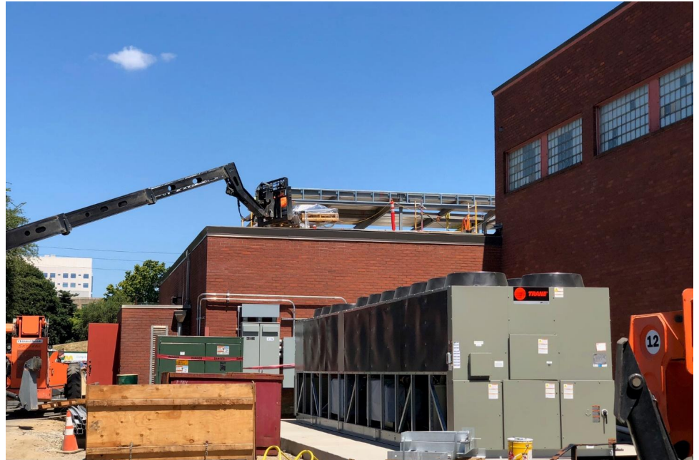
Tubman – New HVAC chiller unit
